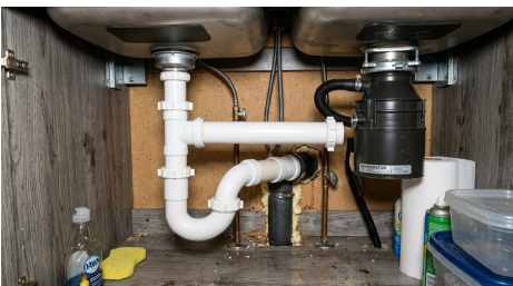
Kitchen sink supply and drain
