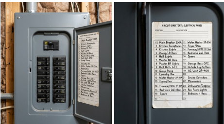
Main panel, labeled
