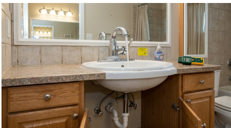
Bath vanity shut-off valves
